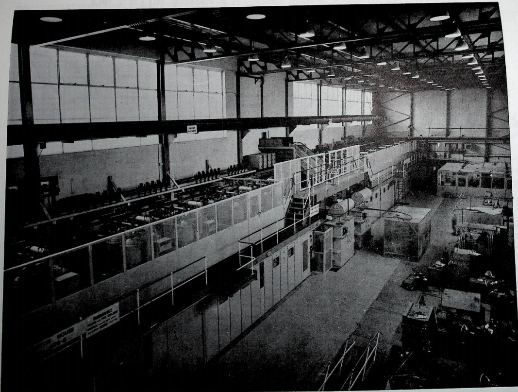
Fig. 5.3.1 (i) View of Converter House showing the rectifier gallery with control gear underneath. The two primary ripple filter chokes can be seen in the centre of the picture and to the right the Brentford regulating transformers.
