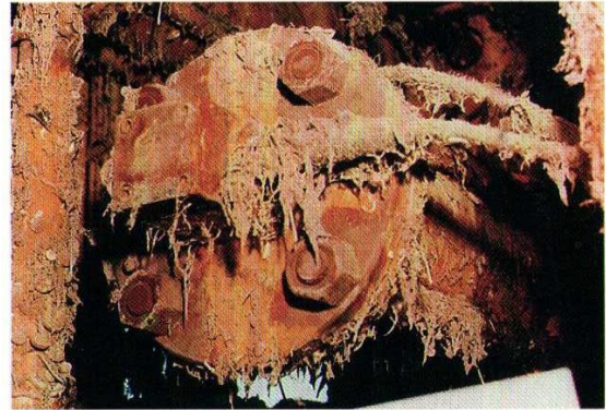
Expertise in seawater corrosion has been compiled as a knowledge based computer system.
