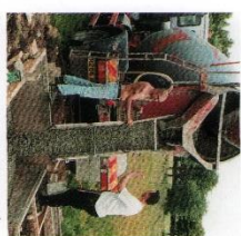
Start of phase one construction work to build the new electrical air station.
