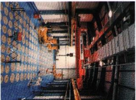
The interim radwaste store where cannot waste is stored in a honeycomb of concrete lined bins.
