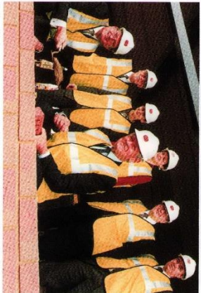
Laying the foundations for new development at the Harwell International Business Centre, UKAEA Chairman, Sir Kenneth Eaton (right) and John Cuts, chief executive, Prologis.
