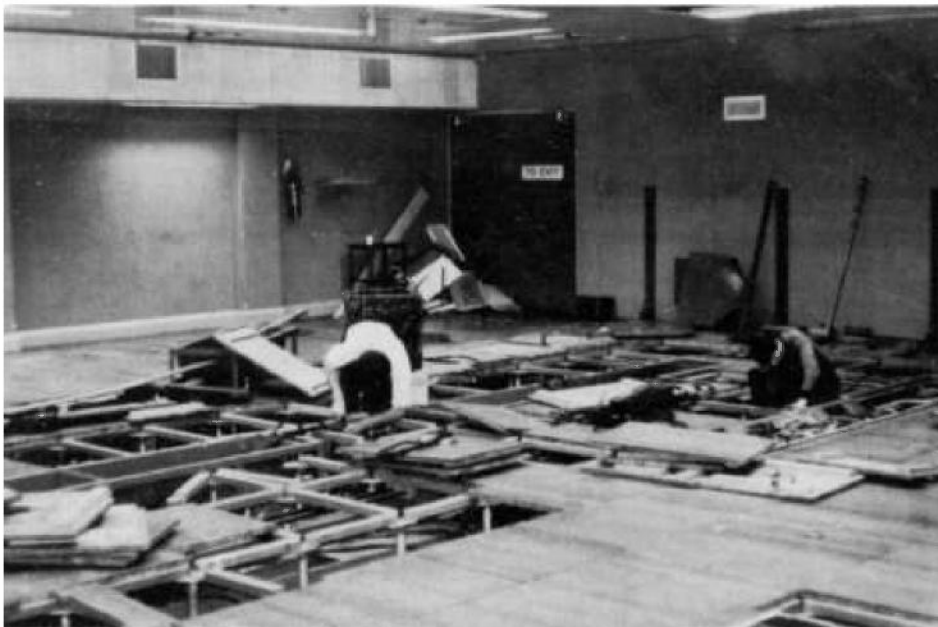
The downstairs room with its false floor, the computer finally removed and the engineers dismantling the cabling of which there was a considerable quantity. Large pieces of cabling had to be of a precise length so as not to upset the timing of the computer's operation.
