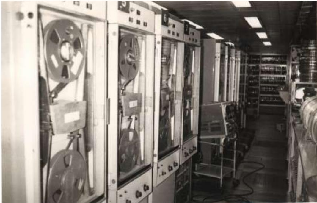
The magnetic tapes were housed in a separate room adjoining the main upstairs computer room.
